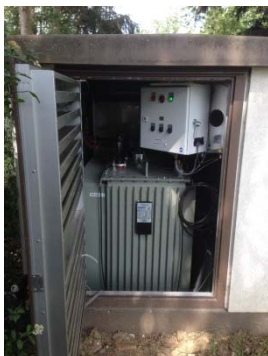
With the type of installation shown here, the transformer connections are safe to touch.
