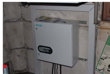
Control cabinet on the right inner wall of the tower substation shown on the left (control cable laid in underground distribution chamber)
