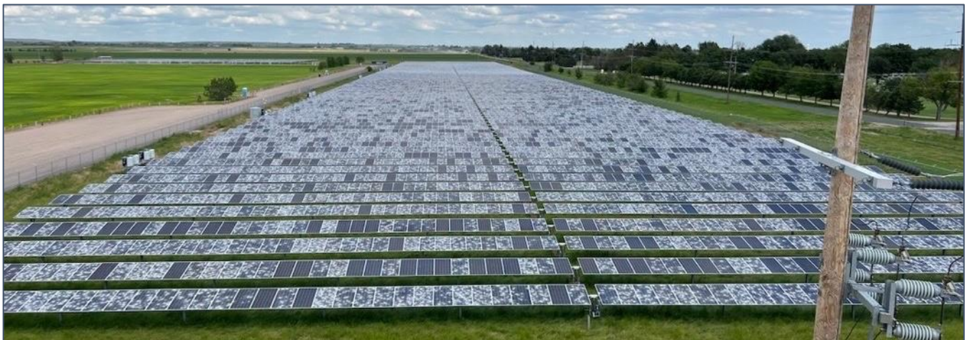
Figure 16. Severe hail damage at a 5 MW Nebraska Public Power District solar project following a June 2023 storm.
